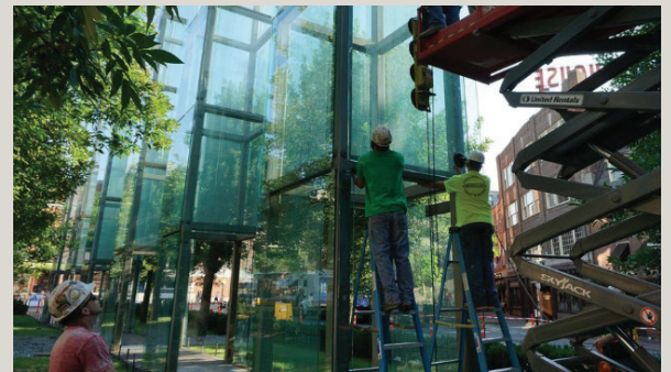
Workers make repairs to the Boston-based New England Holocaust Memorial. Photo: Combined Jewish Philanthropies.
