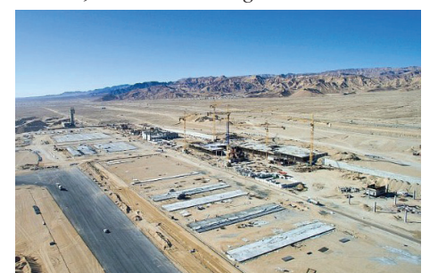
Construction of the new international airport Ramon Airport, which will replace the Eilat airport in southern Israel. Jan. 6, 2016. Photo: Moshe Shai/Flash90.
